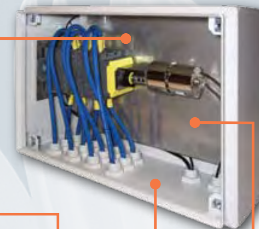
The Emergency Switch
