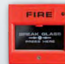
Fire alarm button
